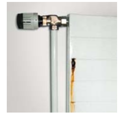
Radiators rusted through
