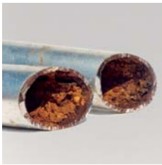
Deposits in the piping
